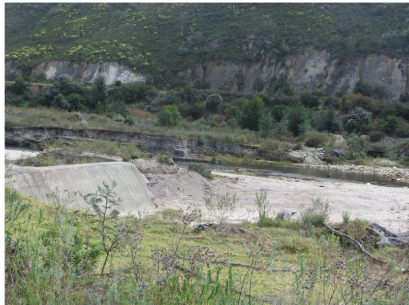
Figure 40: Collapsed gabion Source: Author's work
