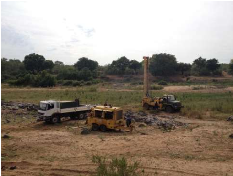
Figure III.1 Drilling river borehole (LRW002) in river bed close to Letaba Ranch gauge
